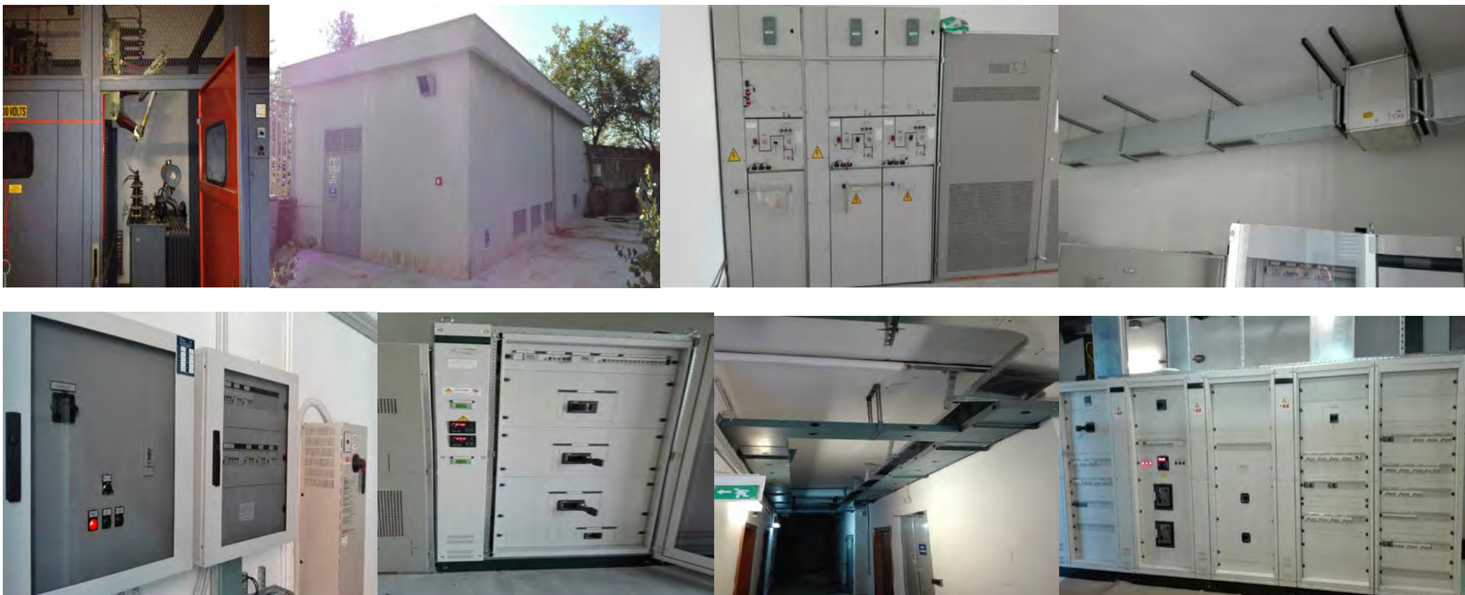
Italy - Battipaglia Belvedere (SA). Interventions on transformer protection and transformer, box trafo group, low voltage panel, automatic power factor correction, main cabin electrical panel, main building electrical panel, cable entry for new connections cables
