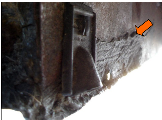
Trunk drop sealant Drain added later
