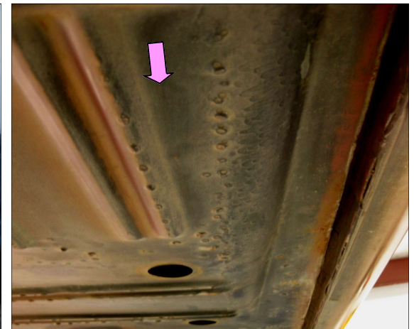
Floor behind rocker lip showing paint shadow.
