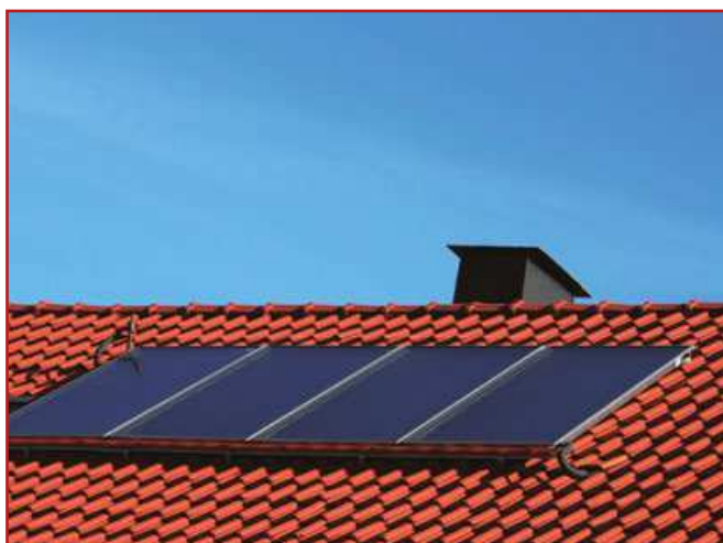
▲ Solar collectors on a roof.
