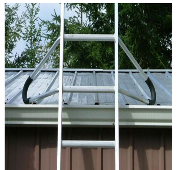
Fall Protection & Fixed Roof Ladders Jamaica, Queens -NY
