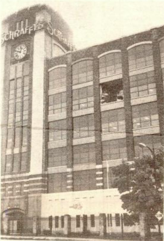
A WINDOW on the fifth floor of The Schrafft Center in Sullivan Square was blown in by the force of the wind during the storm on Friday. The winds were reported in excess of 65 miles per hour. No injuries were reported on this floor, which is occupied by Orion Research.
