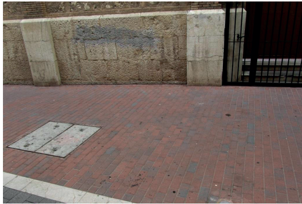
Figure 5: View of the pavement and manhole in Sant Joan de la Creu Street before the rehabilitation of the air-raid shelter, picture by Ivan Cabrera i Fausto.
