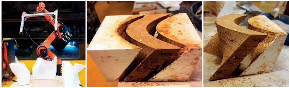
Image 7: The initial experiments with robotic hot-wire cutting EPS blocks and using them as the molds of rammed-earth modules.
