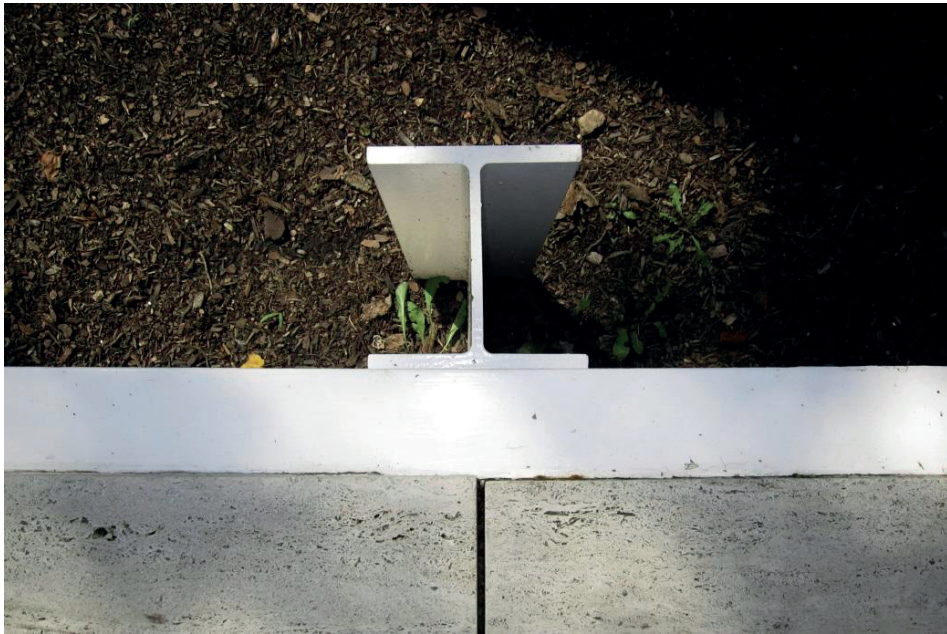
Figure 3: Beam and column junction detail in the terrace of the Farnsworth House, United States, picture by Eduardo Soler.
