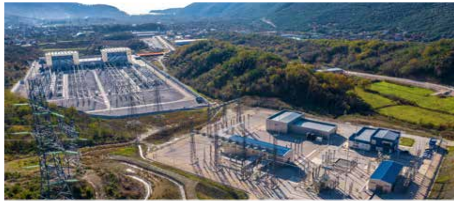
Lastva substation on Trans-Balkan Electricity Corridor in Montenegro completed in 2017.
