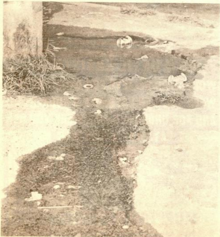
THIS PUDDLE OF WATER is caused by a broken heating line which forces water to the sidewalk surface instead of apartment units.
