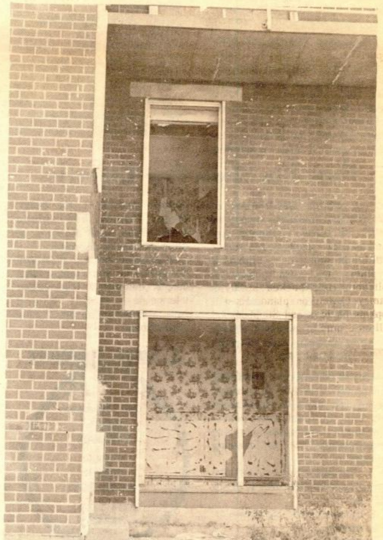
MANAGEMENT LACKS FUNDS to repair this apartment which was abandoned because of defective workmanship and materials which allow water to pour in during a storm. Vandals also have left a mark of broken windows and damaged walls.
