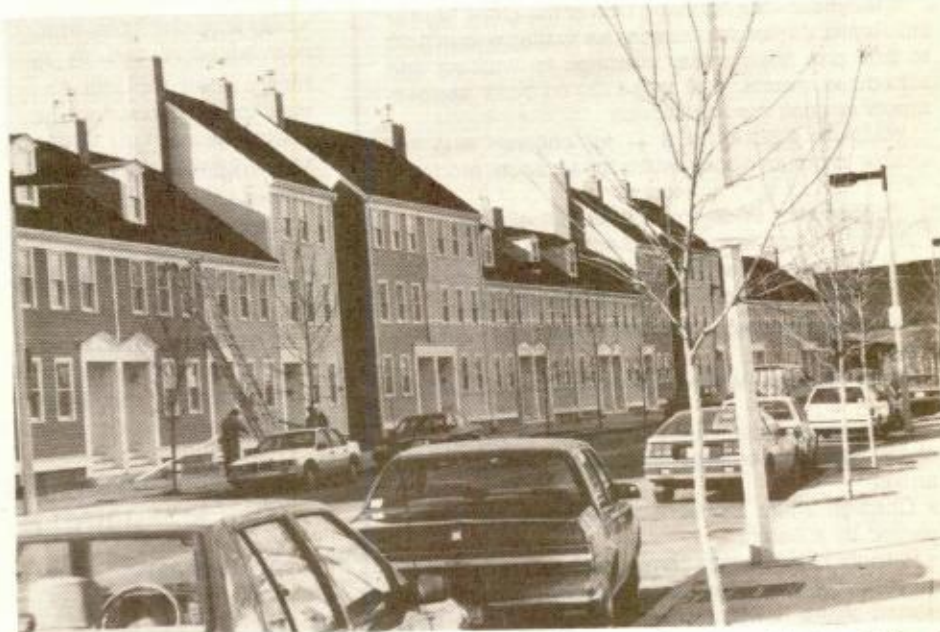
FINISHING TOUCHES are made on the Main Street Townhouses, and the development's construction timetable is well ahead of schedule.
