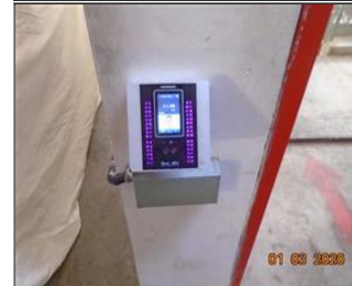
Photo of the inside of the main production hall Time keeping system.JPG
