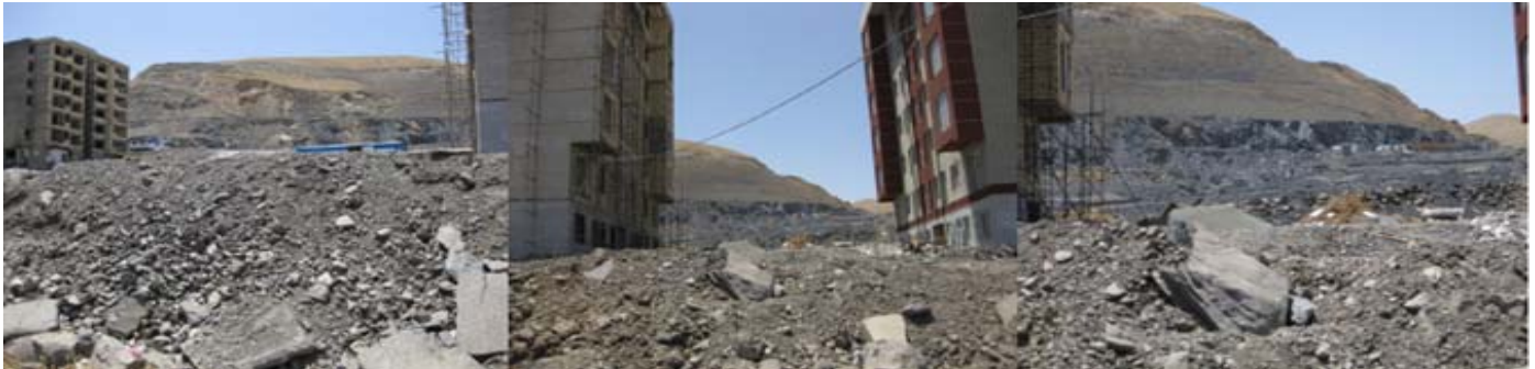
Fig-7: Prevention from inside-to-outside view and including view toward Abidar Range- Huge size excavation and destruction of hard mounts
