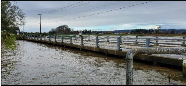
Bridge at risk of floating during high water conditions
