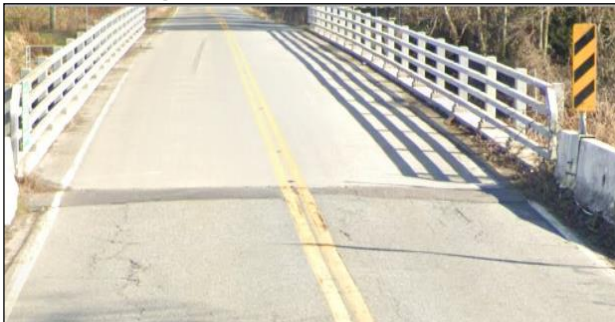
Bridge Deck & Approach Deterioration
