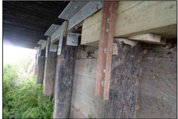
Deteriorating bridge abutments
