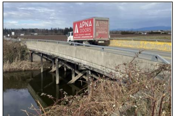
Bridge Deck & Approach Deterioration
