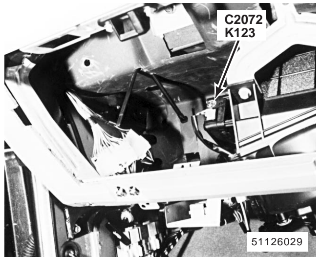
100. behind LH side of fascia K123 Air Recirculation Solenoid C2072 (4-Y)
