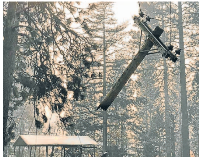
A utility pole was heavily damaged during last year's Camp Fire.
