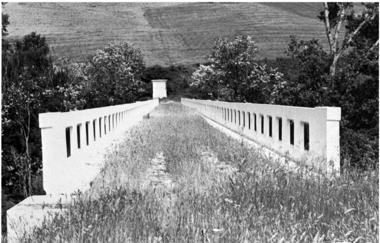
The Tragino aqueduct as it appears today. The water runs in a hollow duct beneath a grass surface which allows it to be used also as a bridge. It was repaired within two-and-a-half days, and
