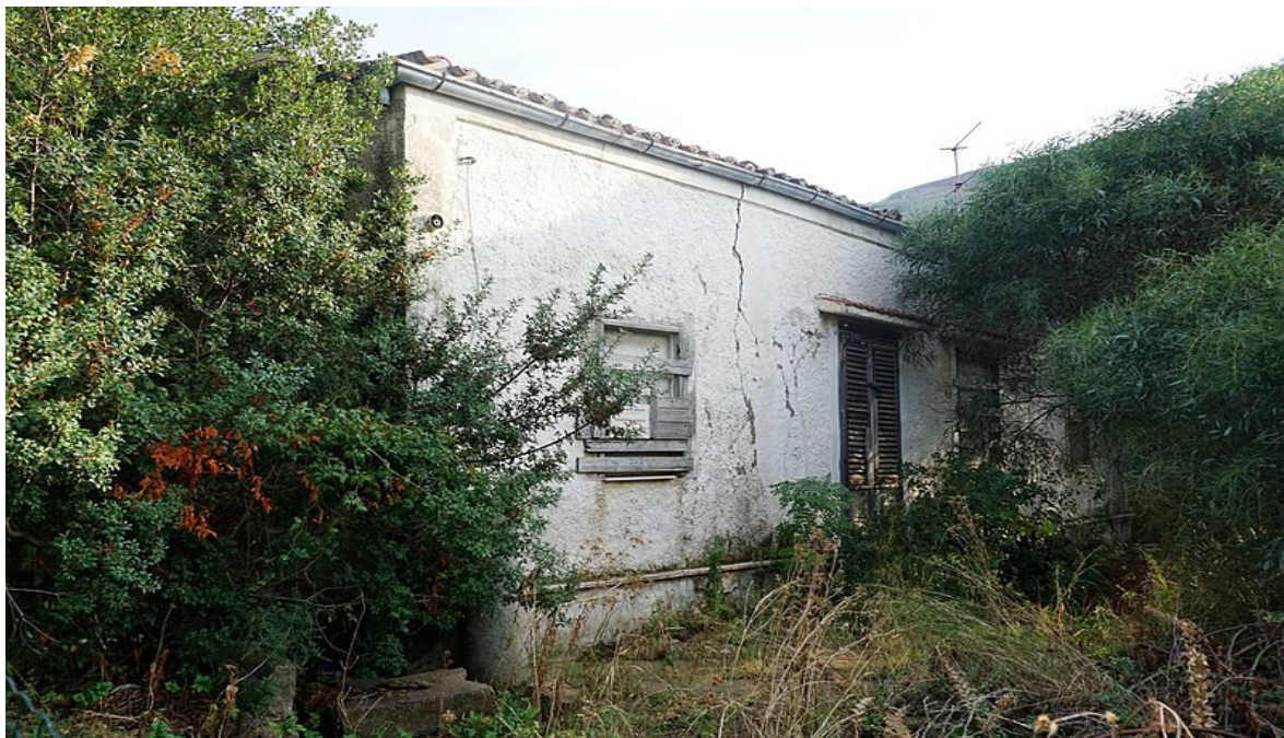
The dilapidated Abbey of Thelema in 2017
