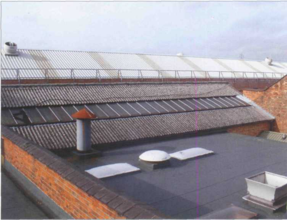
Figure 2.57 Complex roof area with examples of roof lights, fragile surfaces and barriers providing collective protection.
