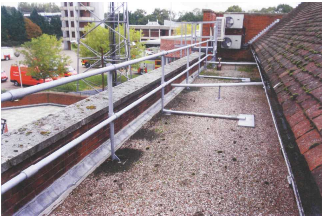
Figure 2.56 Example of edge protection retrofitted to a flat roof to prevail falls from height.
