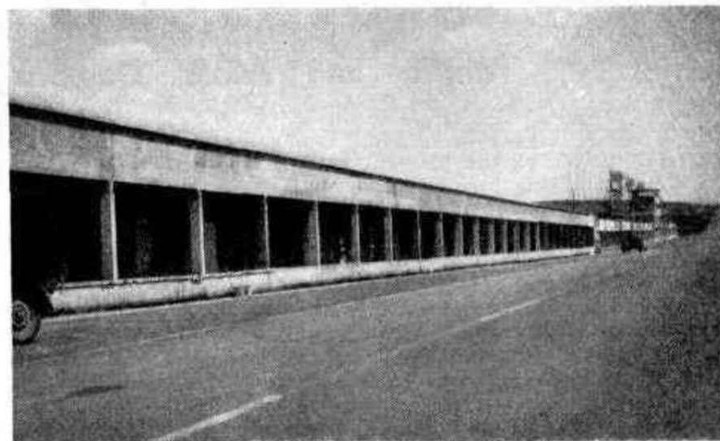
ELBOW ROOM. —In the past the 12-hour sports-car race at Reims has suffered from a large entry and not enough pits; now 30 new concrete pits have been constructed, extending the line right up to the Dunlop bridge on the brow after the start.
