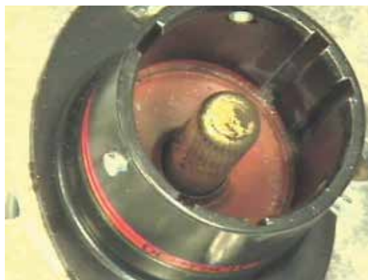
Figure 3: Black fretting marks on this contact are one of the earliest indicators of vibration damage
