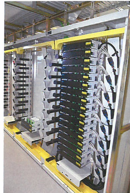
Exhibit 9-6: Example of Cabinet Install
