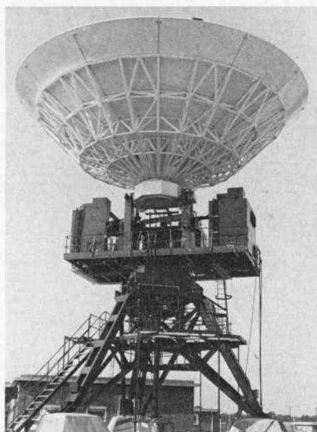
Skynet master communications terminal
