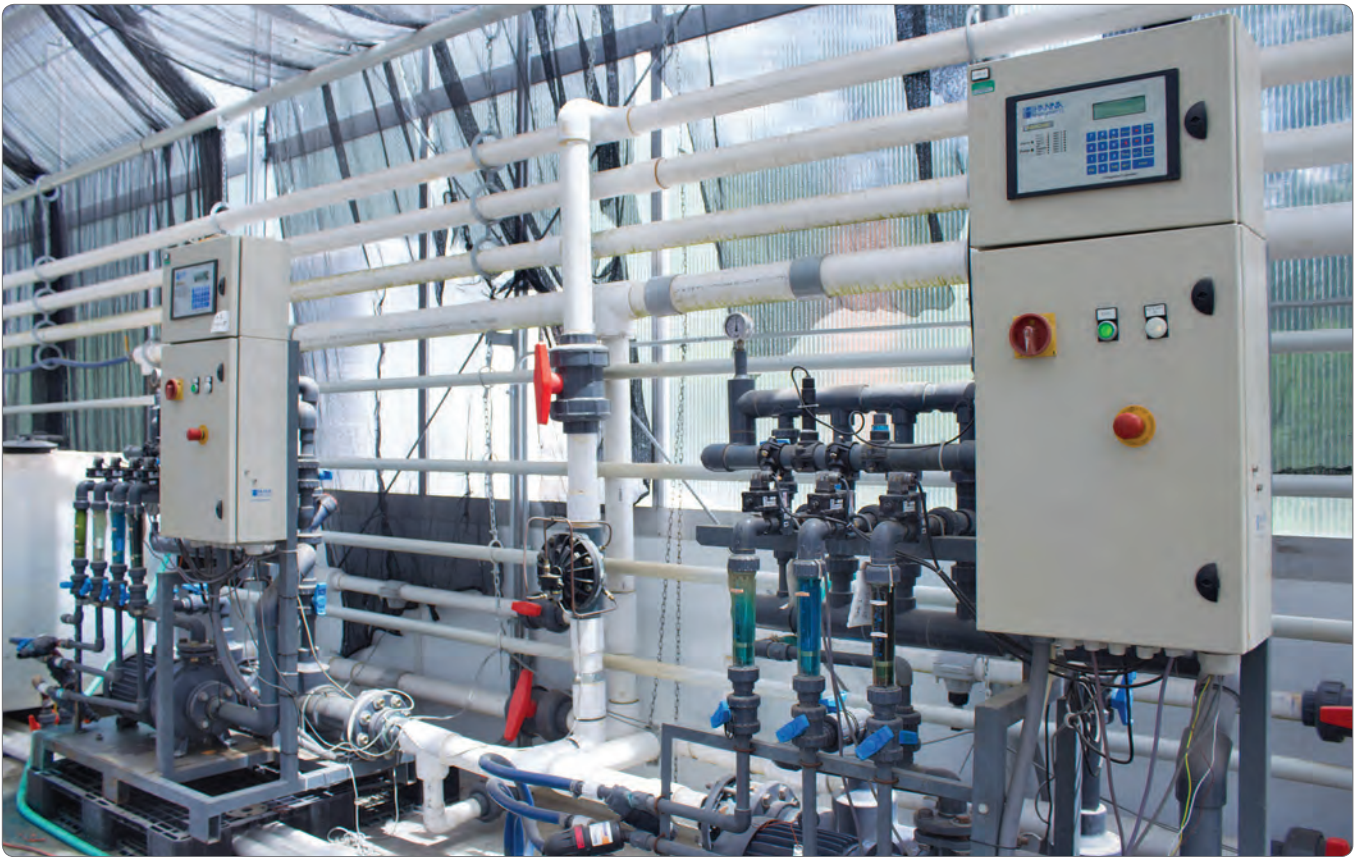
Two panel mount units used in a fertigation system
