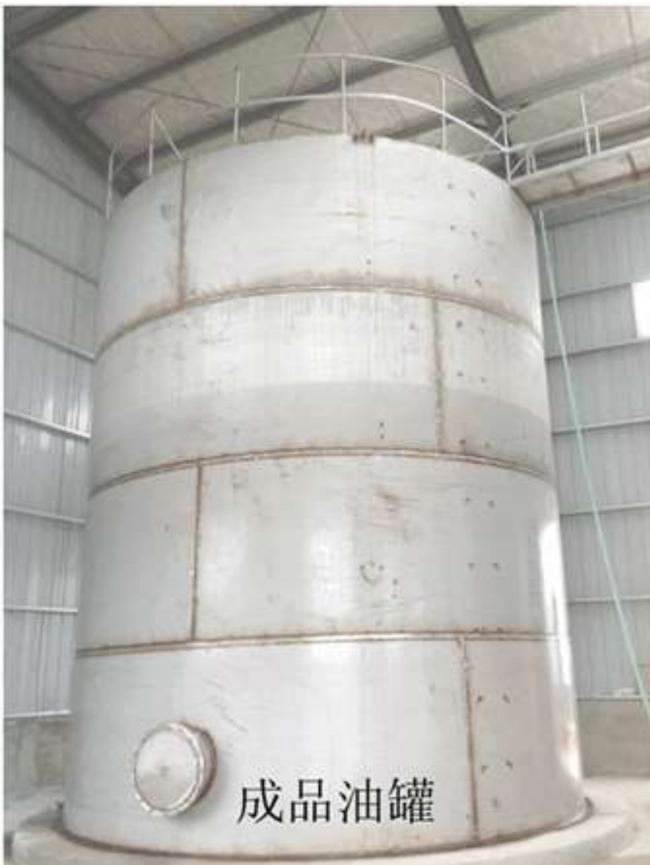
Finished product oil tank
