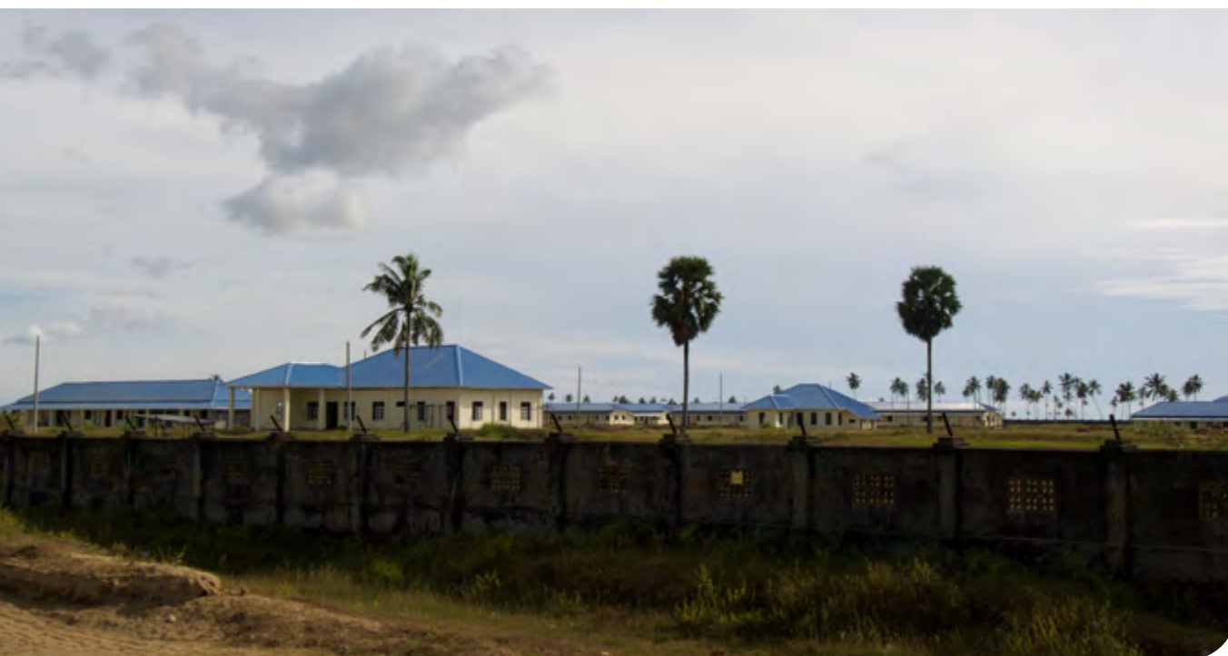
Police buildings under construction adjacent to Rohingya detention camp complex, Sittwe, December 2014
