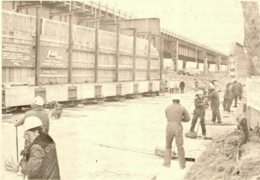
INCH BY INCH workers of Alar Corporation operate winches, steadily moving the over 100 year old wall to line up with the wall visible in the upper right hand corner of the photo.
