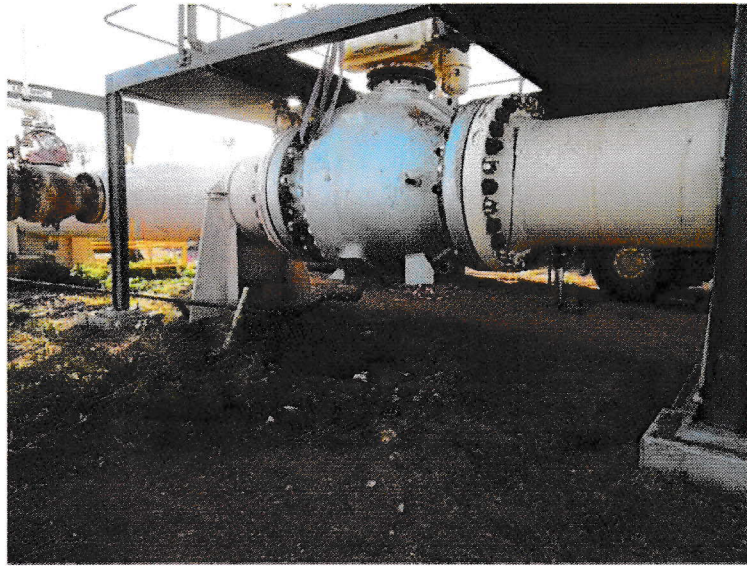
Photo 1: Isolation Valve at Toolachee Trunkline Pig Receiver
