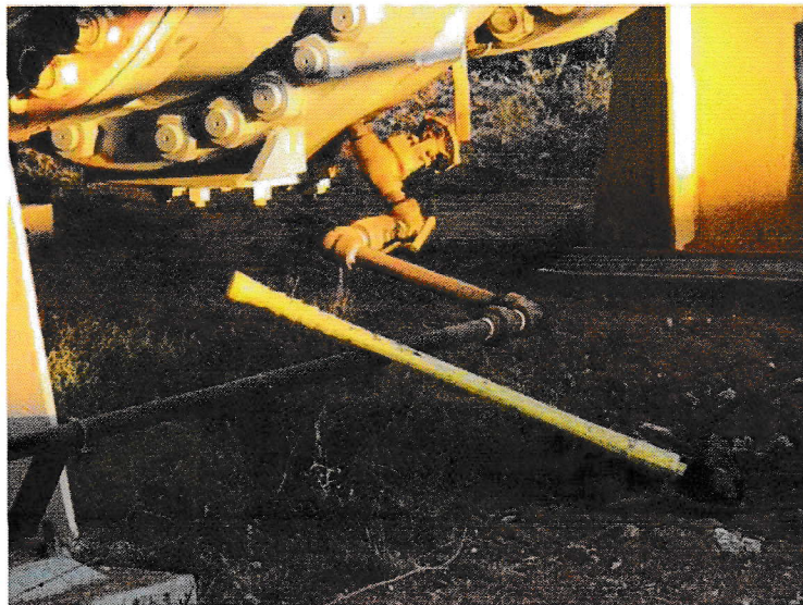
Photo 2: Dropped object (sledge hammer) on valve cavity drain line
