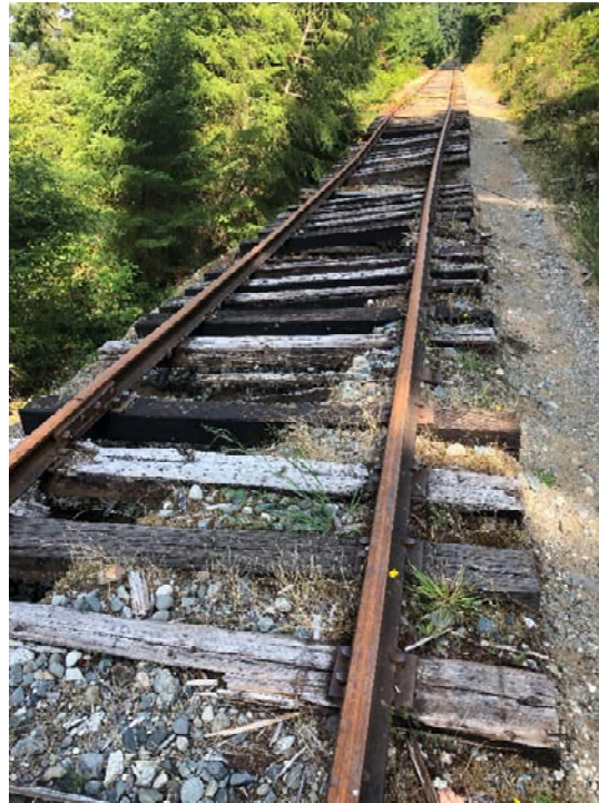
Figure 8: Slope Failure at mile 22
