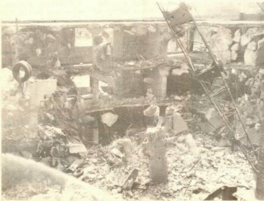
ONLY A SHELL remained last weekend as the former site of Cataldo's garage on Warren and Park Streets was demolished by the wrecking ball to
