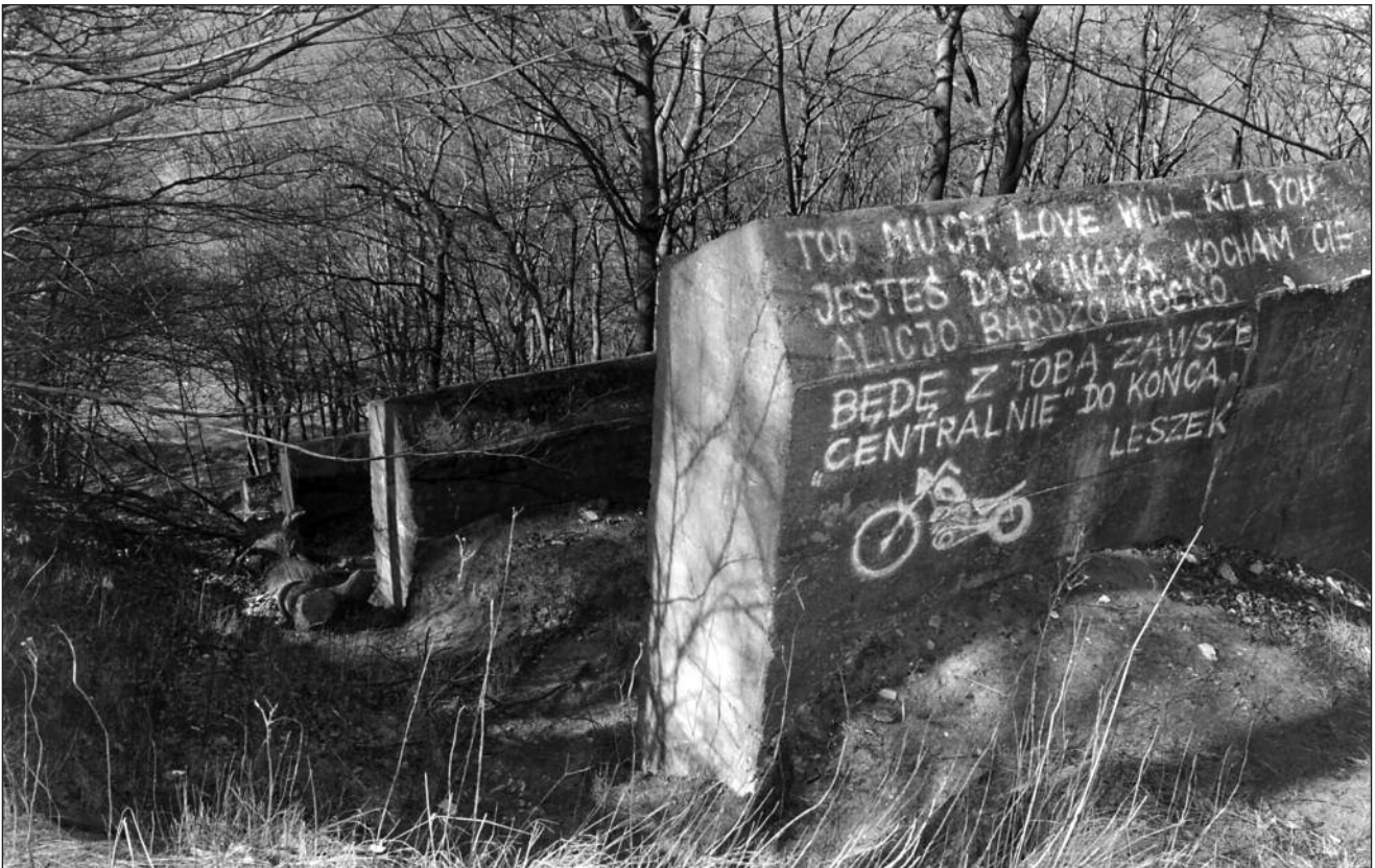
This is the series of nine concrete supports that carried the upper part of the second ramp (see page 7). When compared to what had happened to the first ramp (see top), the foundations appear to have been of better quality here and none of the supports had given way. Another 100 metres down the road,
