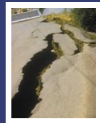
Many highways and roads could be made impassable by cracks and landslides following an earthquake.
