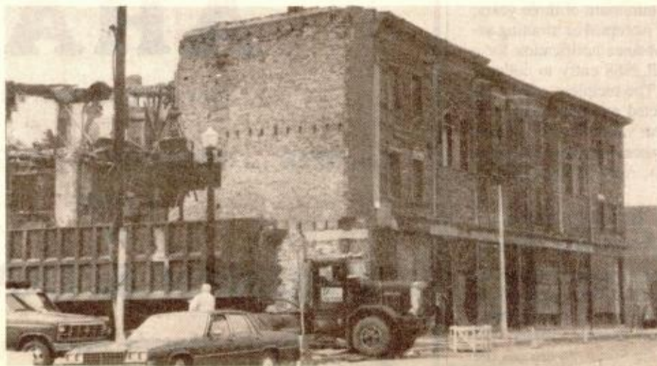
DEMOLITION is underway at the former Liberty Bell Wholesale Grocer's building on Main Street to make way for 26 new town-houses, including 13 affordable units, being developed by the Charlestown Economic Development Corporation. (photo by Kathy Giordano)
