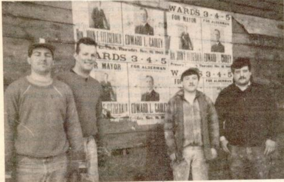
WORKMEN renovating the building at the corner of Bunker Hill and Monument Streets uncovered political posters on the building's wall under the layers of cement and shingles that created the building's facade. Shown (l. to r.) Jacko Greatorex and John Dowd of Charlestown, and Martin Ward and Stephen O'Brien originally from Dublin, Ireland.
