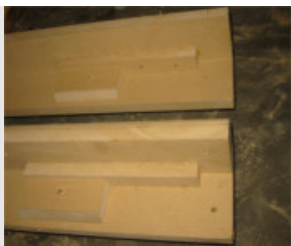
On the inside of my corner posts I fitted some spacers on one side which the side-walls would butt up against, on the front edge I put some wider blocks which extend out to where the door meets the post and they had a slanted edge
