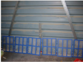
A row of windows ready to go – there's quite a sense of achievement in getting a pile like that together.
