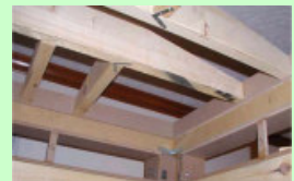
You can see the bracing affixed to the box frame section of the upper roof
