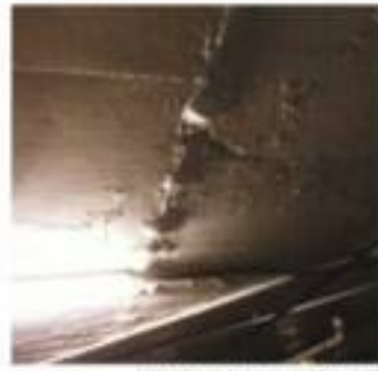
This photo released by Surfside, Fla., in a 2018 report shows cracking on floor slabs in the garage at Champlain Towers.
