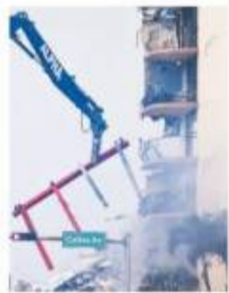
Debris removal was hampered by fires burning underneath.
