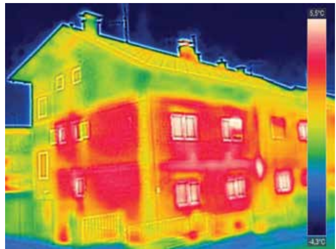
Figure 3.5. Thermal imaging of a home shows where heat is being lost. The red colour indicates a higher temperature which means those areas of the house are losing more heat to the outdoors. The yellow and green areas of the house are better insulated and lose less heat.
