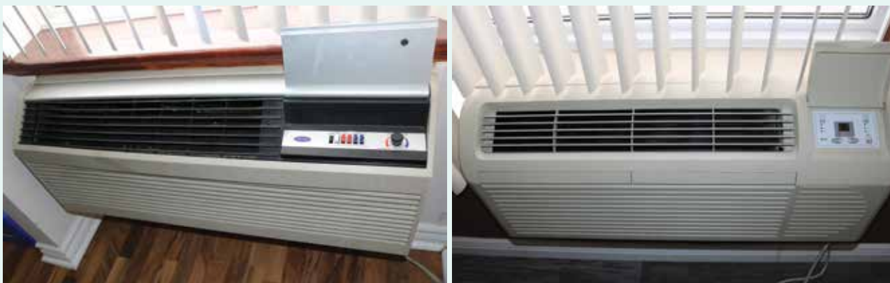
Old air-conditioning unit (left) at the Peninsula Inn Hotel in Niagara Falls switched for an energy efficient packaged terminal heat pump unit (right) under the pilot.
