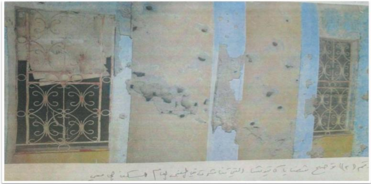
Katyusha missile effects on the building of the university accommodation
