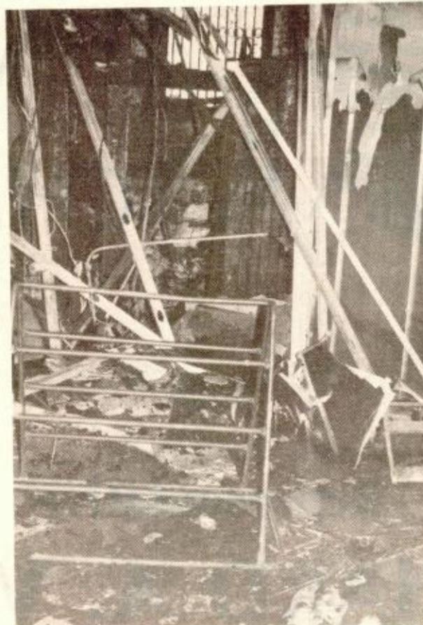
CHRISTMAS PRESENTS for the Headstart children had been stacked in this basement room and set on fire. (photo by Kathy Giordano)
