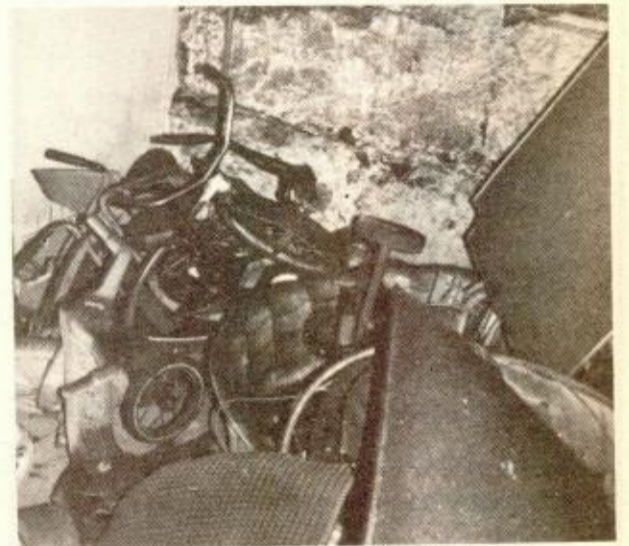
TOYS AND EQUIPMENT for the Headstart program lie in the corner of the basement, stacked and burned by the arsonist. (photo by Kathy Giordano)
