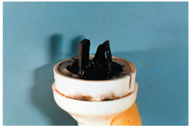
FIGURE 19.24 The 3-pin plug. The extreme heat has melted the plastic center causing the pins to deviate from their normal vertical positions.
