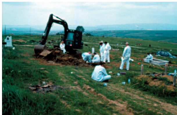
FIGURE 28.16 Removal of top soil from a proposed mass grave in a cemetery on the outskirts of Pristina, Kosovo.
