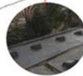
Aesthetically poor roof and canopy
