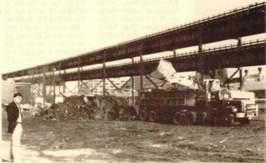
DAVID FLANAGAN, community liaison for MDPW, overseeing the removal of debris from the BHA owned parcel of land in Hayes Square that was being utilized by a contractor for MDPW in the CANA roadway reconstruction project. (photo by Kathy Giordano)
