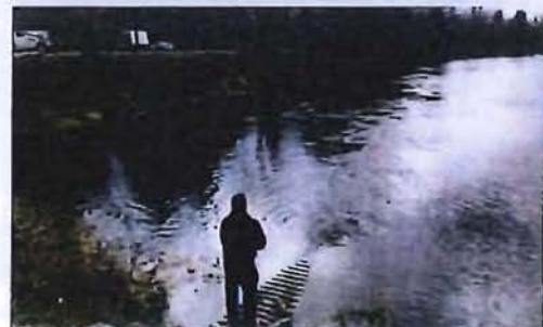
Figure 3-12: Surcharged culvert servicing private driveway
