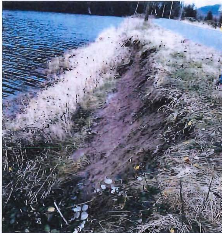
Figure A-3: Section of Seabird Island Road embankment sloughing - approximately 10 m long
