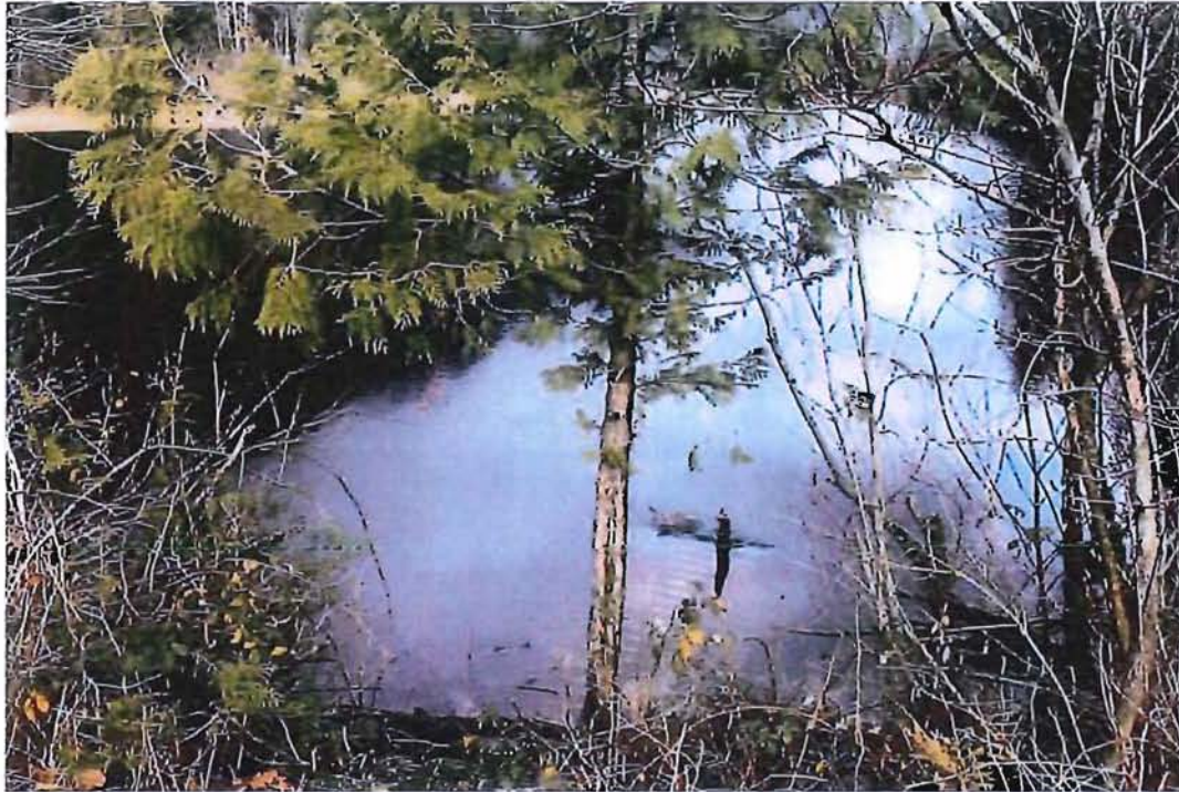
Figure A-23: Surcharged culvert servicing private District of Kent driveway. Site 05D
