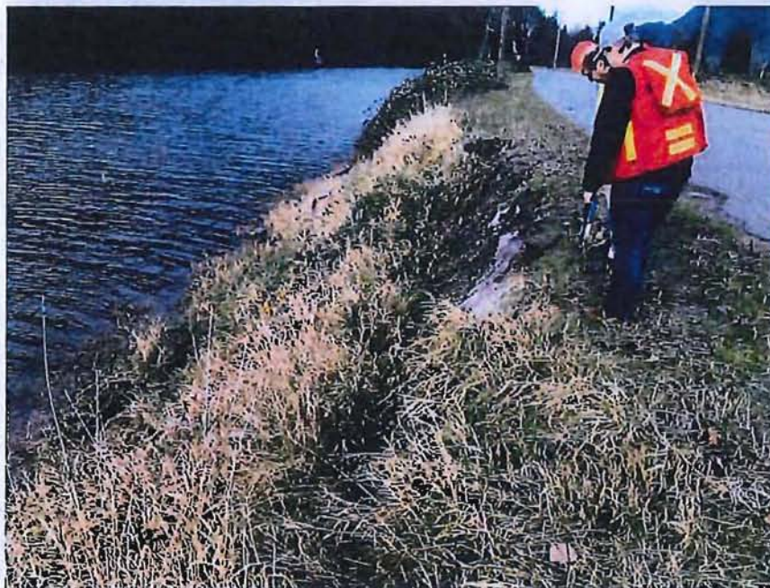
Figure A-2: Tetra Tech staff measuring sloughing section along Seabird Island Road
