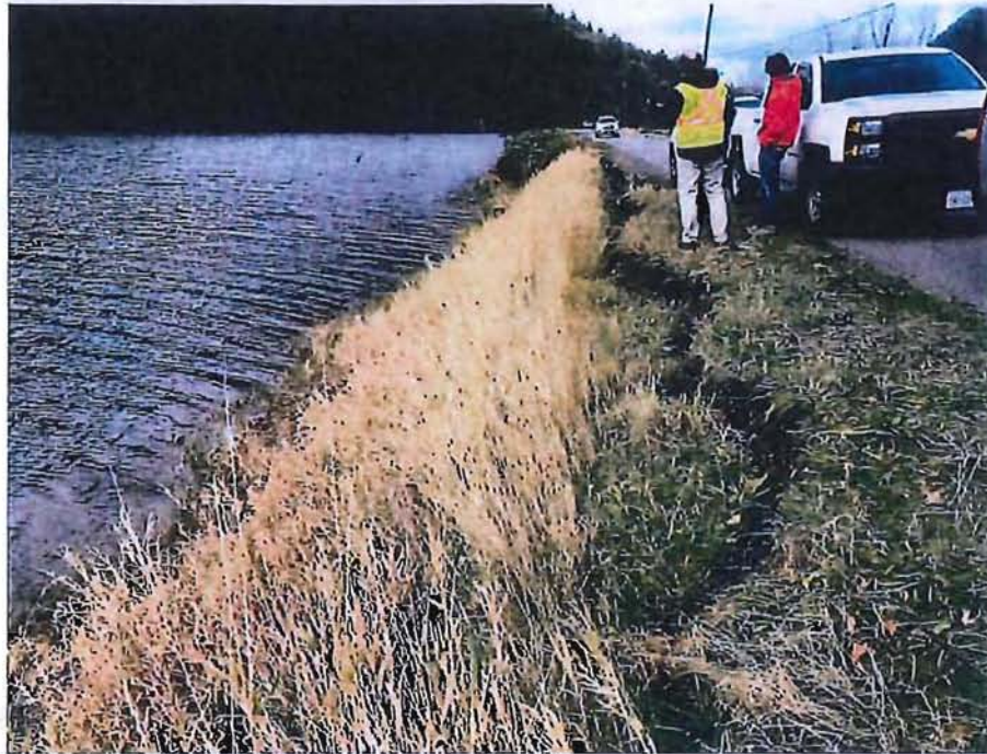
Figure A-1: Section of Seabird Island Road embankment sloughing - approximately 50 m long
