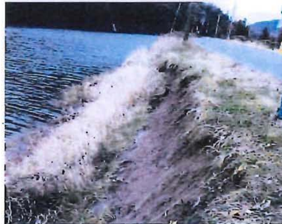
Figure 3-2: Sloughing on the west side of Seabird Island Road
