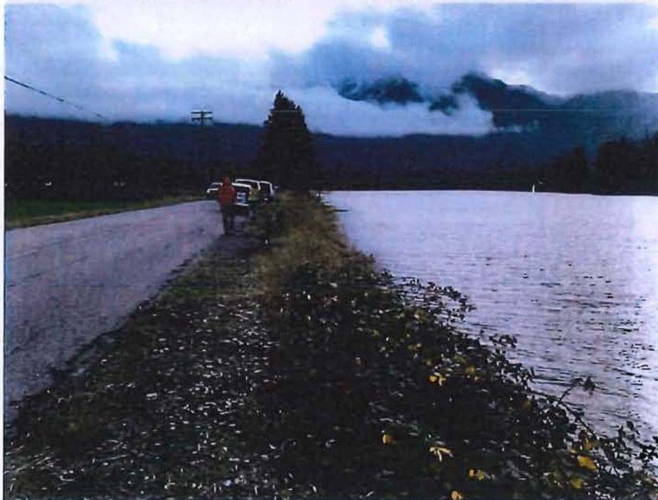
Figure A-4: Sloughing section along Seabird Island Road
