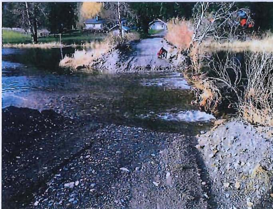
Figure A-22: Deconstructed private access road intentionally overtopping during field visit. Site 05D.
