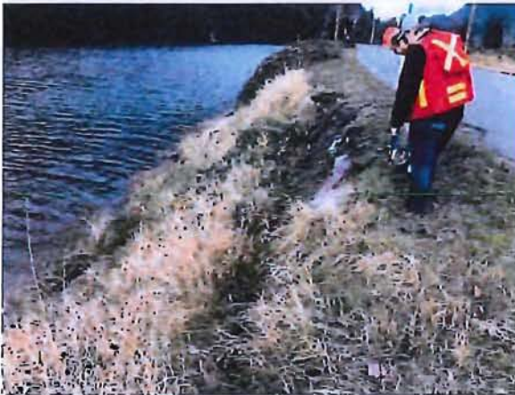
Figure 3-1: Tetra Tech staff measuring sloughing on the west side of Seabird Island Road
