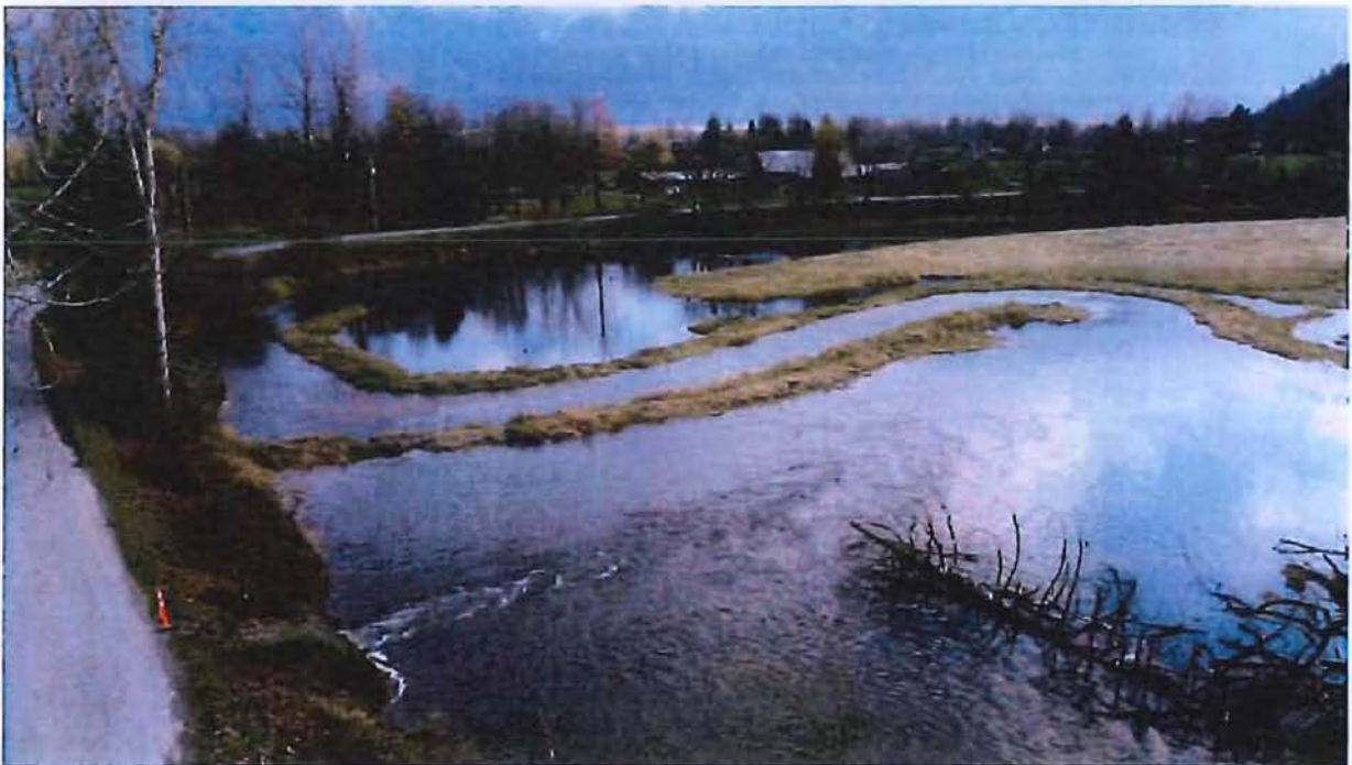
Figure A-24: Aerial view of failing wood stake culvert crossing site. Site 05B.
